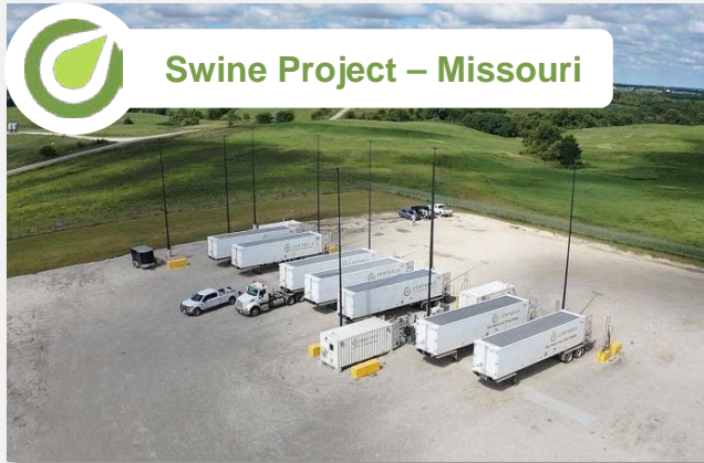
Injection site servicing four swine farms in northern Missouri
