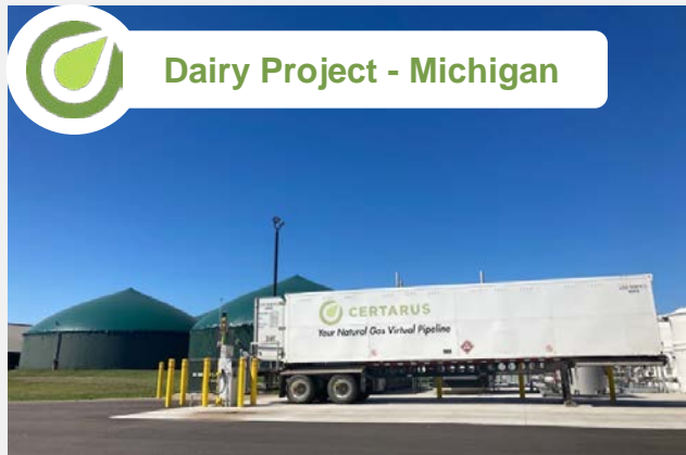
Recent announcement of first gas off dairy digester project in Western Michigan
